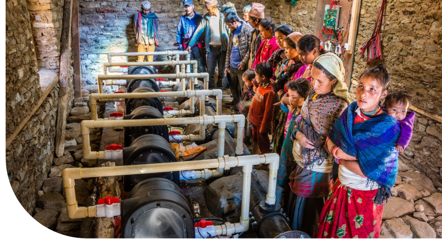
Pico-hydro turbines working with VS and Xtender in Nepal
