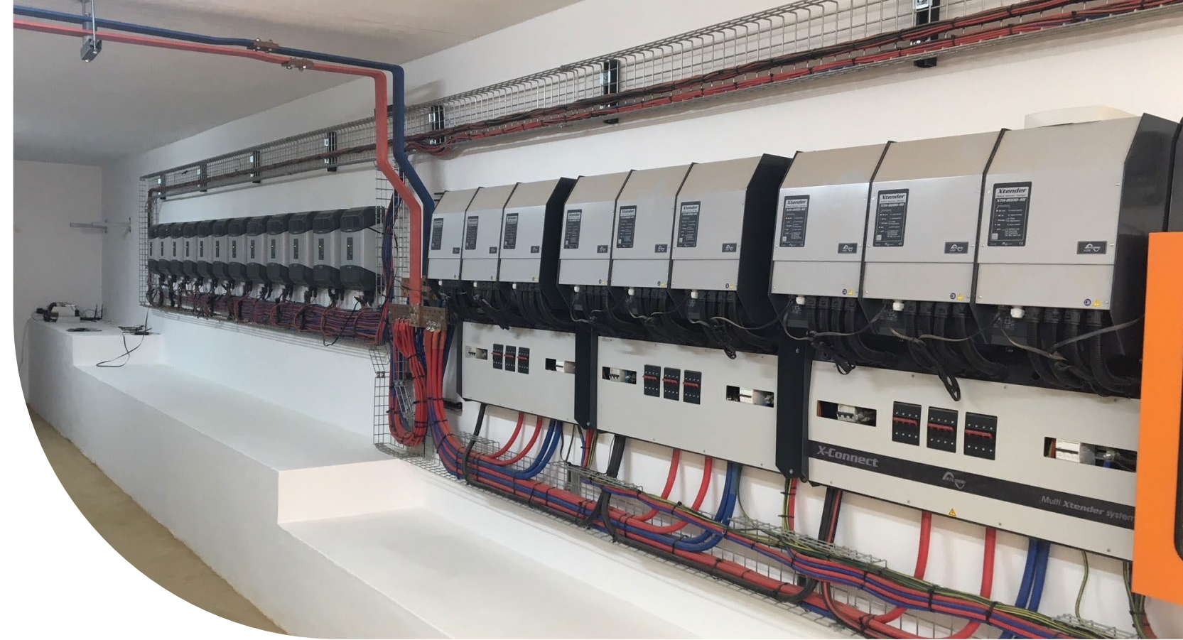
72kW hybrid offgrid system in South Africa
