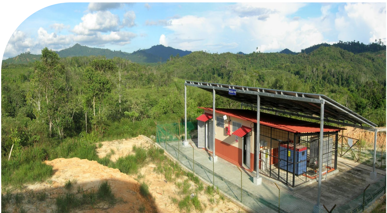
Hybrid systems for a school in Malaysia
