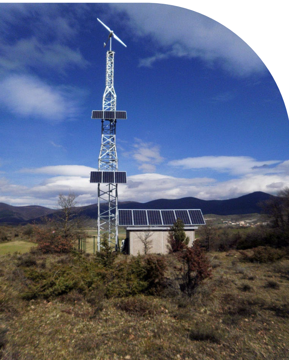
Itelazpi offgrid telecom tower, Spain
