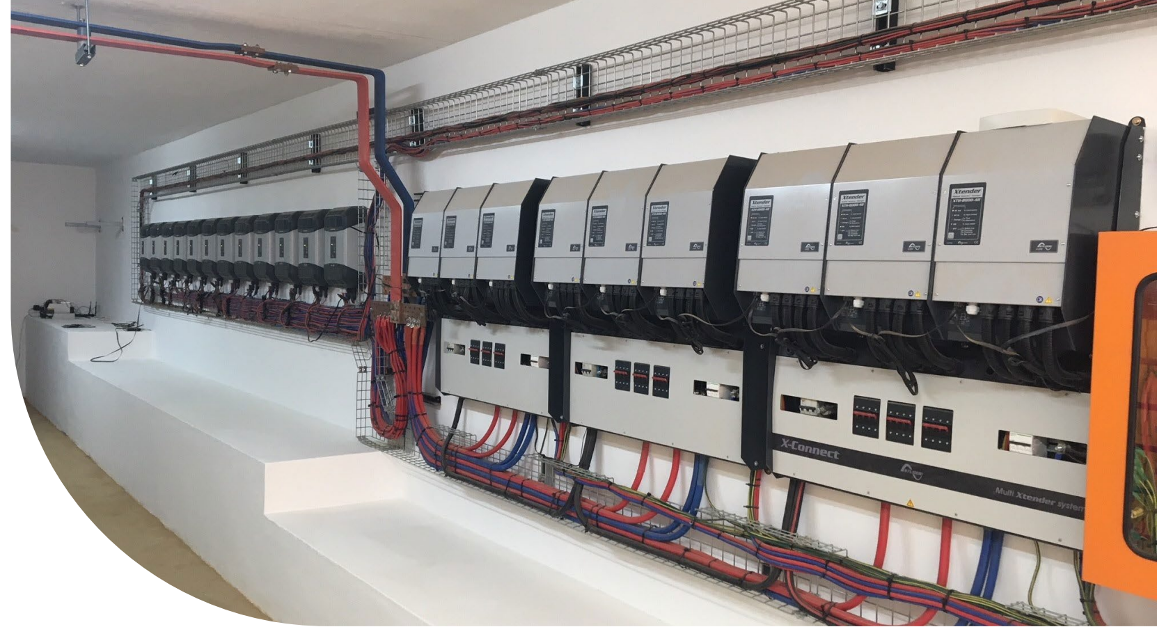
72kW hybrid offgrid system in South Africa
